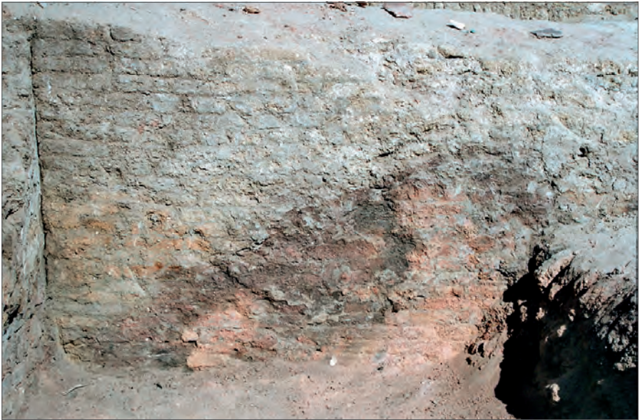
Fig. 20. Burnt patch on the western face of the east wall of Room AA.50.4, view looking east (Photo W. Godlewski © PCMA)
