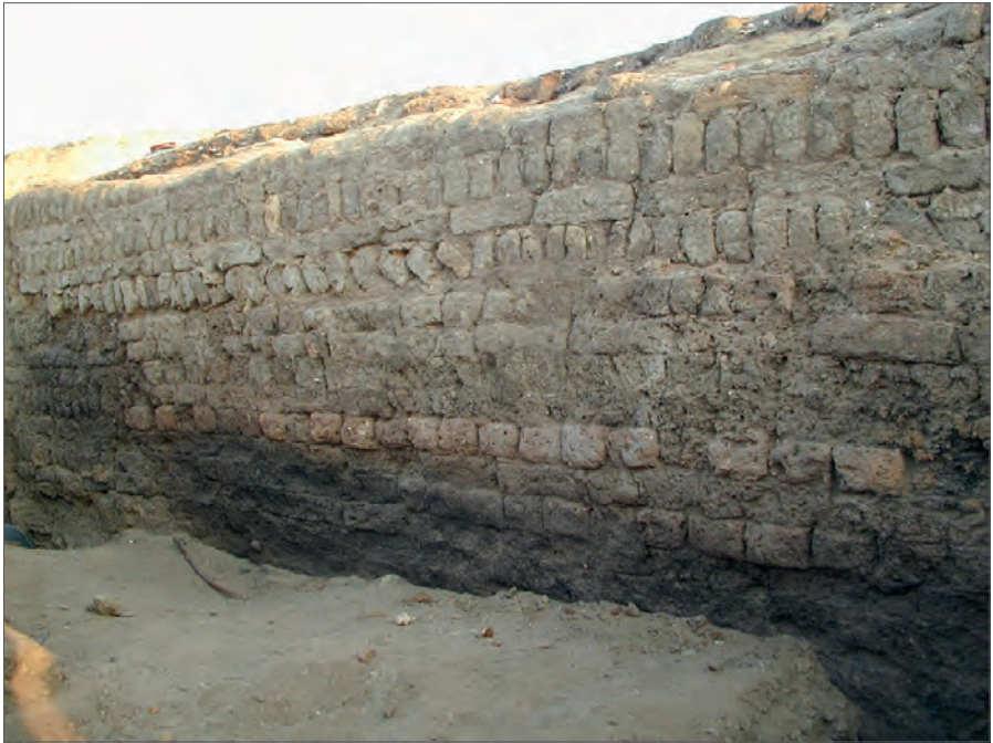
Fig. 22. Traces of burning on the northern elevation of Building J, looking southeast (Photo W. Godlewski © PCMA)
