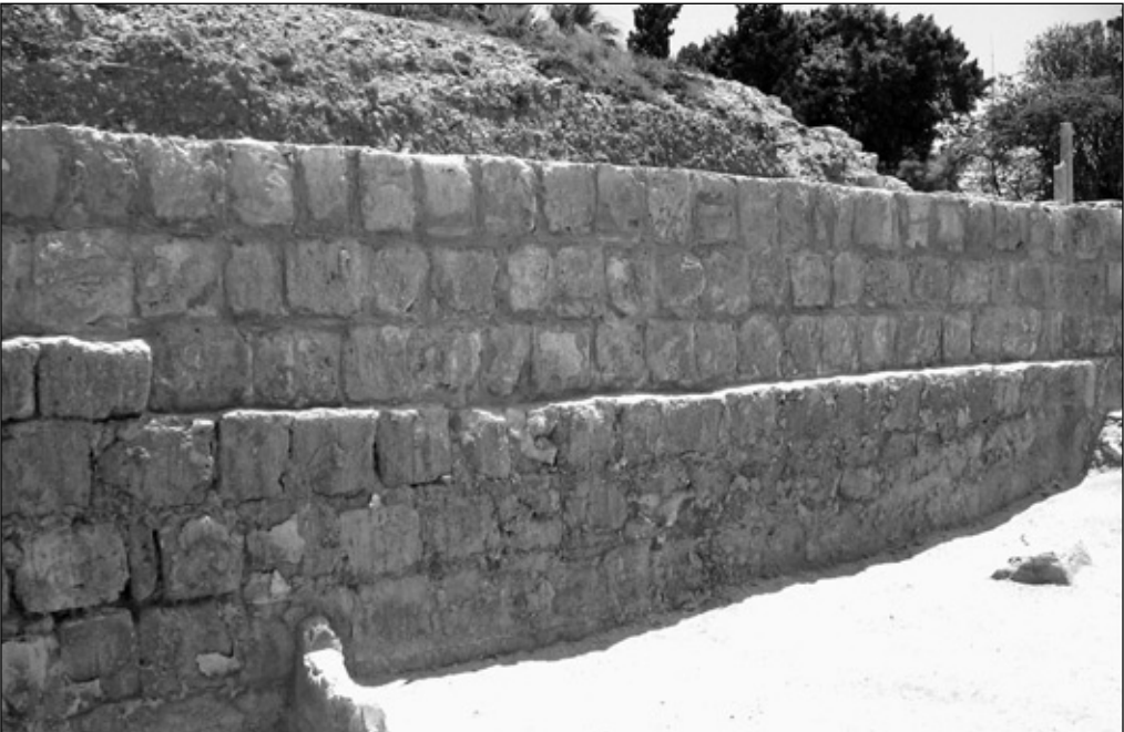
Fig. 8. Auditorium L, eastern wall before (top) and after consolidation (Photo G. Majcherek)
